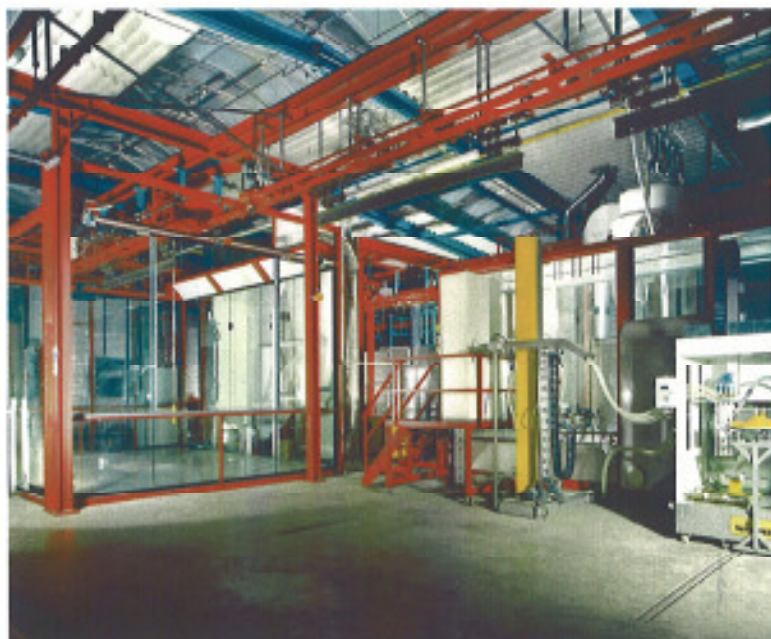
Powder coating machine with preliminarily operated RÖSLER shot blasting machine
